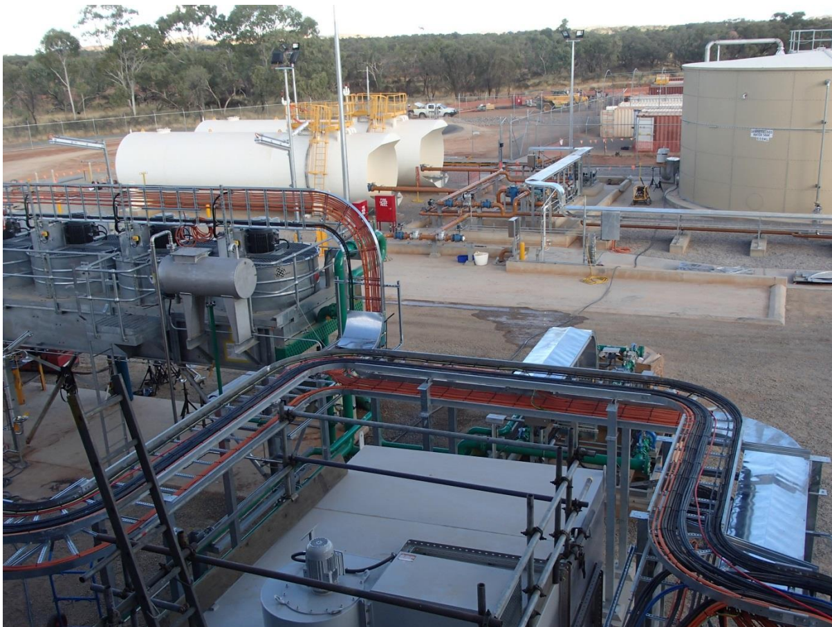
LV Electrical Installation Leichardt Power Station – Leighton Contractors
